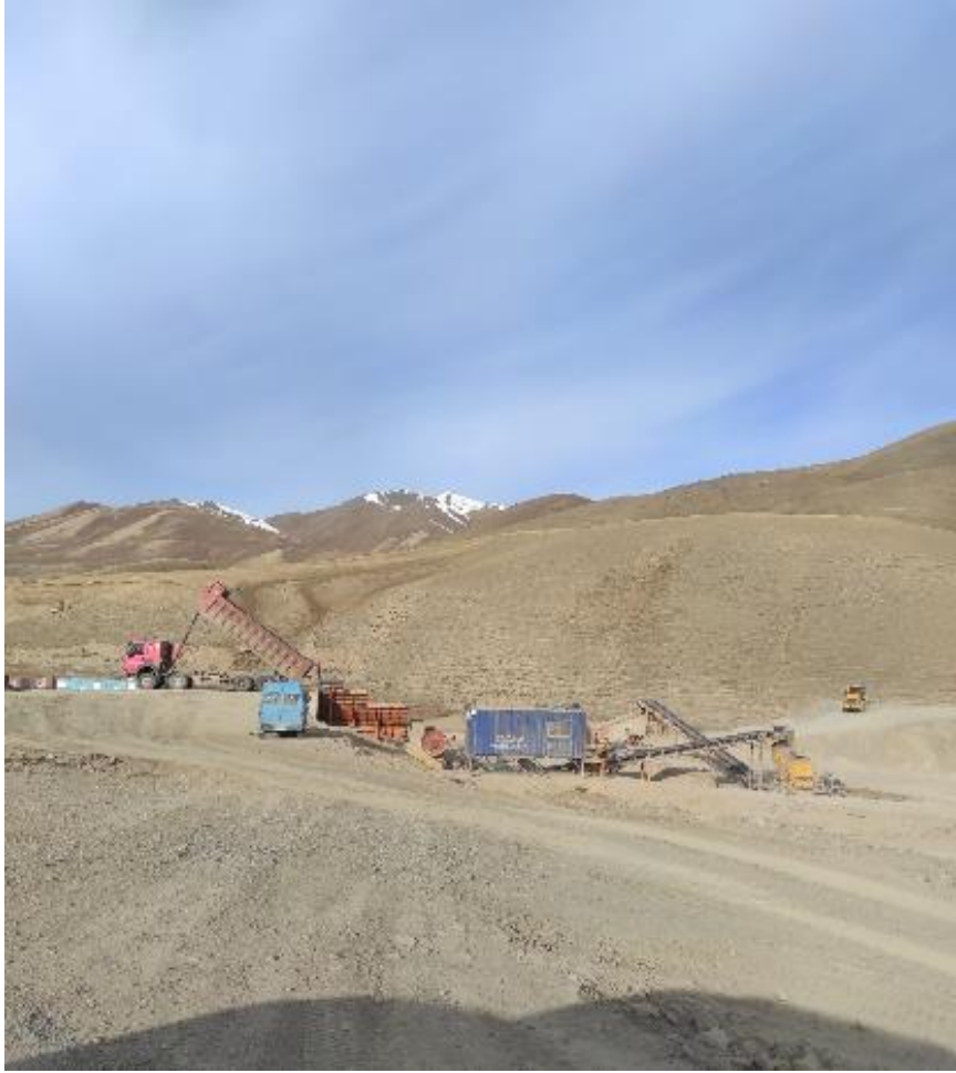
Figure 21: Crusher at the production site (km 106+300).
